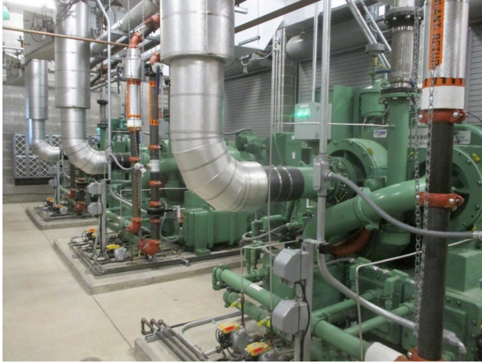
Photo II-3: Air compressors for the Soo Locks to service air bubblers (Richard Stewart)
